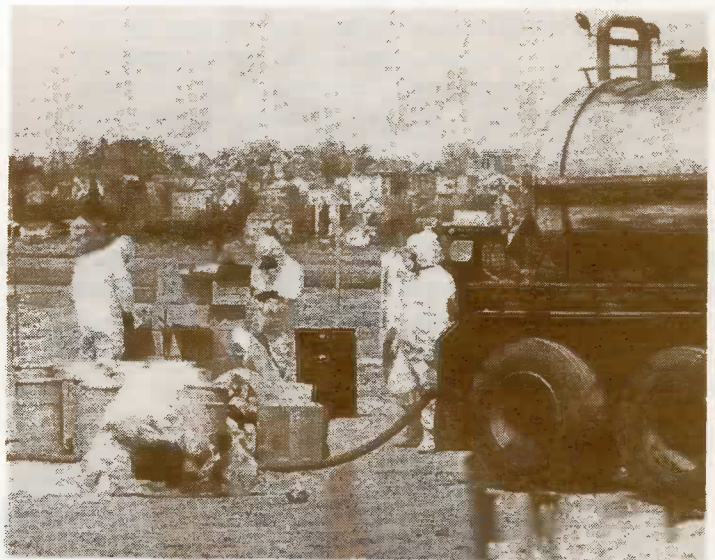
Protective clothing and masks were needed to pump out Methyl Methacrylate from the barrels safely.
